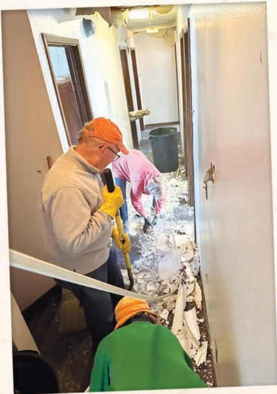
What a difference! The Trust's early cleanup efforts following damage from a burst water line.
